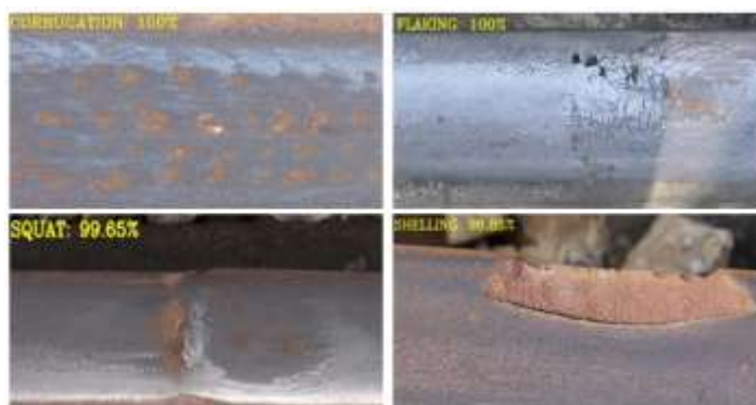
Fig. 7. Detected Faults in Railway Track
